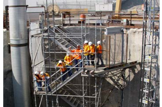
ESD 112 students tour the "Big Pipe" project by Impregilo/S.A. Healy in Portland
