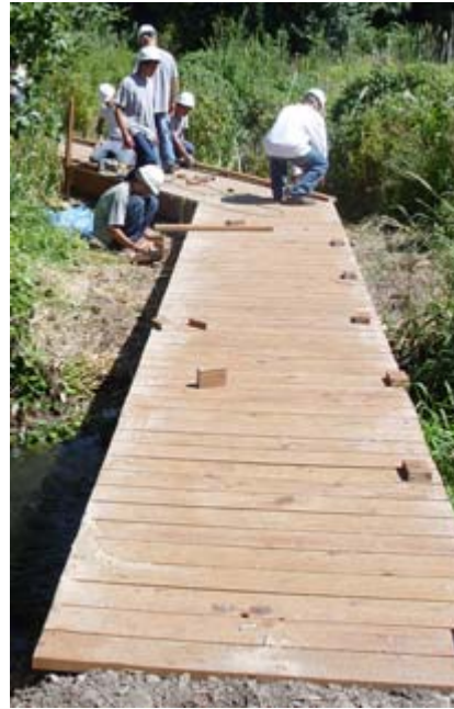
A little math, a lot of measuring, and the walkway heads in the right direction.
